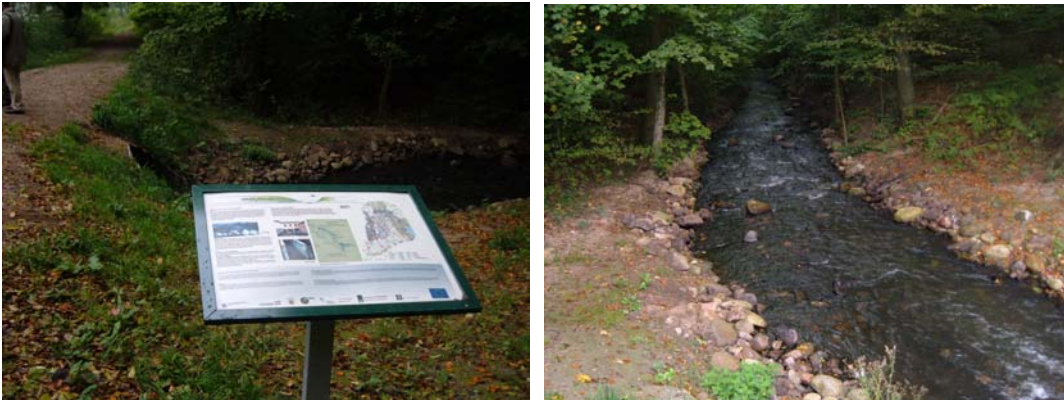
Left: An interpretation panel close to the diversion channel. Right: the man-made diversion channel looking downstream from the lake outflow. Boulders have been placed to provide flow variation and armouring.
