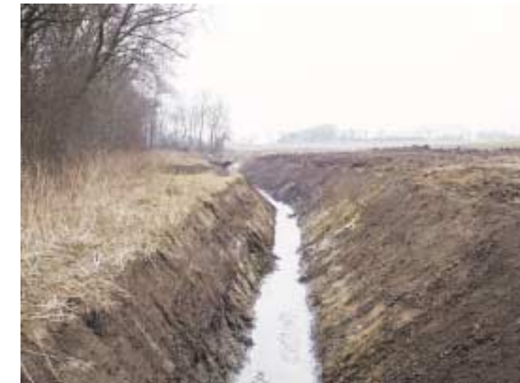
Sand migration in a small watercourse because of heavy-handed maintenance
