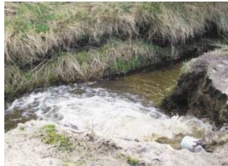
The drain has washed the bank away
